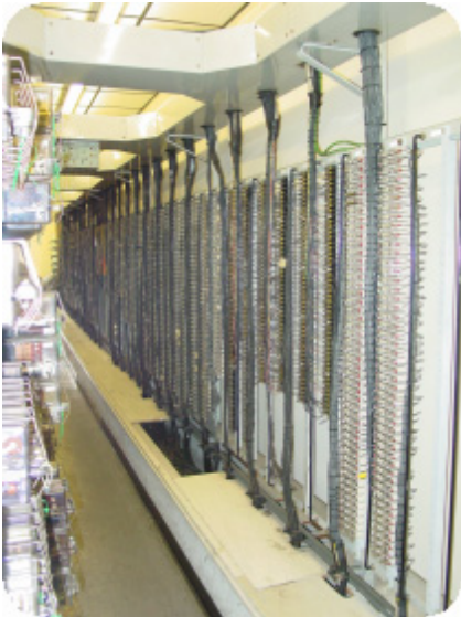
Central relay room
