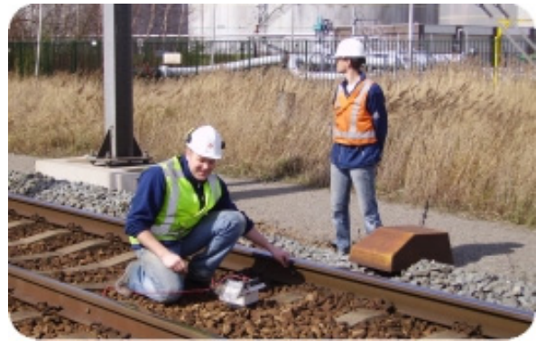
Set up Jade safety system
