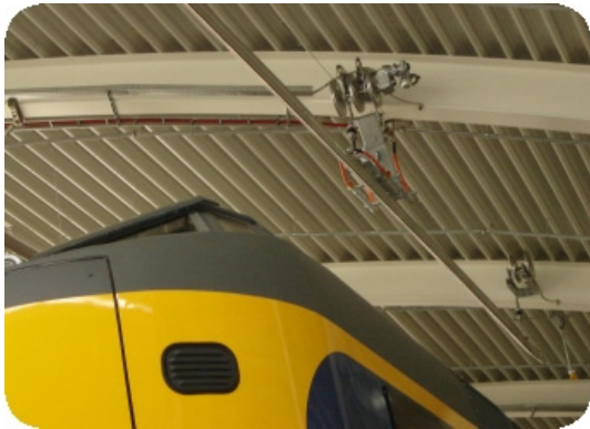
Movable catenary systems
